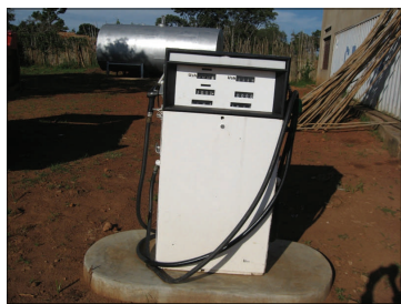
Fuel Tank ready and waiting to be filled with fuel
