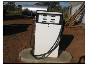
Tank and pump installed and ready to be filled
